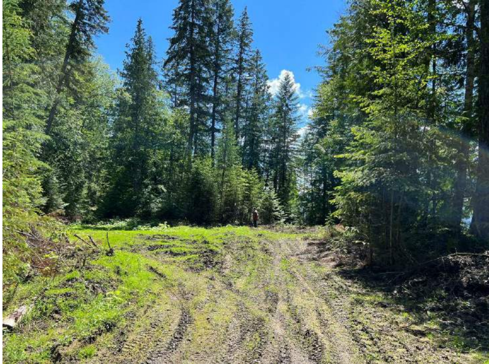
Plate 10-1: Collar for drillhole C97-12 from which holes D22-01 to D22-03 were drilled
